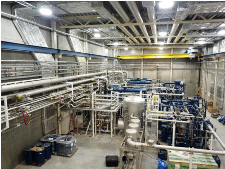
Compressor system at the European Spallation Source Accelerator Cryoplant in Lund, Sweden
