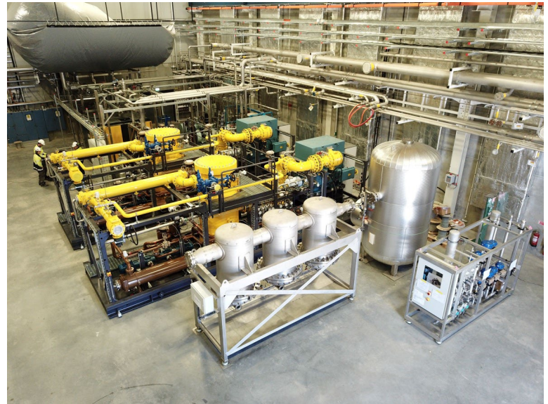
Compressor system and oil removal skids at the European Spallation Source Target Moderator Cryoplant in Lund, Sweden
