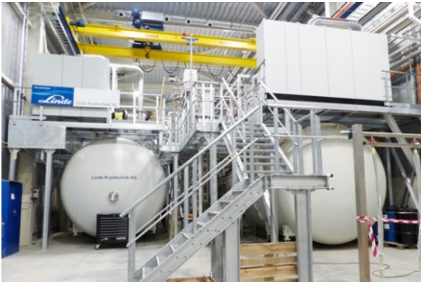
Cryoplant cold boxes at the European Spallation Source Accelerator and Target Moderator Cryoplants in Lund, Sweden
